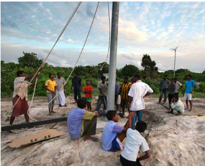
The Skystream towers were raised without the benefit of heavy equipment. Villagers young and old lended their time to the effort.
