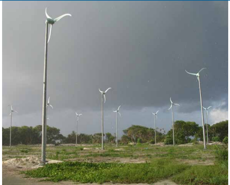
A site with 24 turbines at Haa Alif Uligamu (Uligam) island in the Maldives northern atoll.
